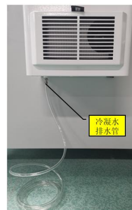
Figure 68: Condensate Drain Pipe of Air Conditioner
